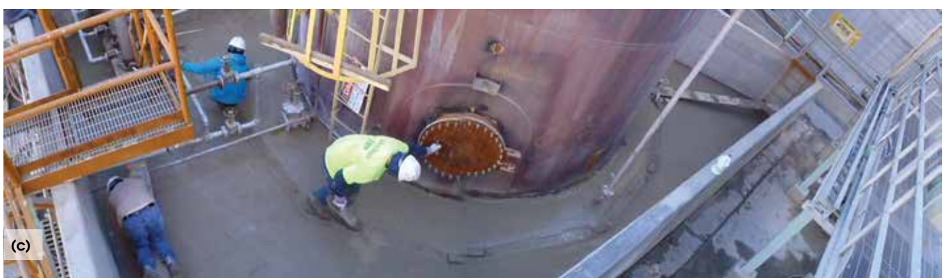
Fig. 3: TOPCOR Services workers construct a containment slab near a sulfuric acid storage tank: (a) damaged concrete on the existing slab was removed, and reinforcing bars were placed for the new containment slab; (b) the activated fly ash cement concrete was mixed and delivered using conventional equipment; and (c) it was finished using conventional methods
