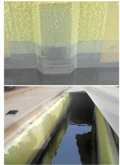
KEMROK Cement Concrete Sulfur Trench After 2 Years of Service (No Degradation)
