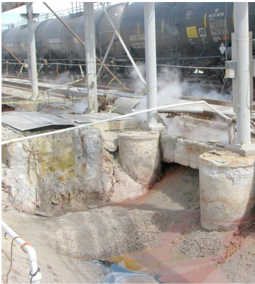
Deteriorated Portland Cement Concrete Sulfur Trench
