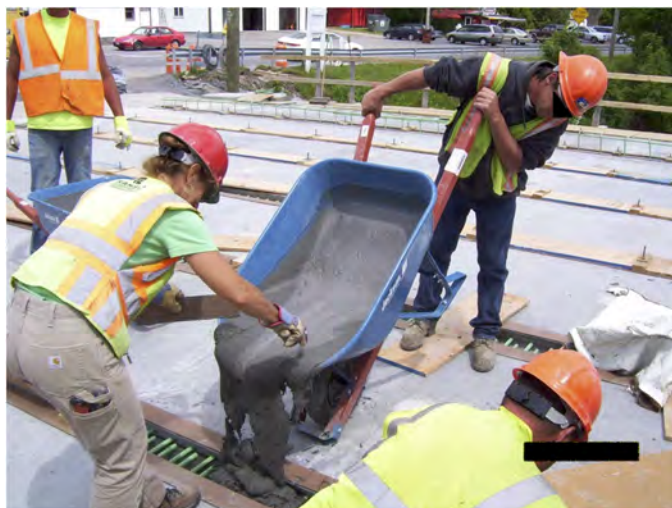
Fig. 1. Longitudinal connections between the top flanges of two deck-bulb-tee prestressed concrete girders being cast with UHPC (reprinted with permission from New York State Department of Transportation)
