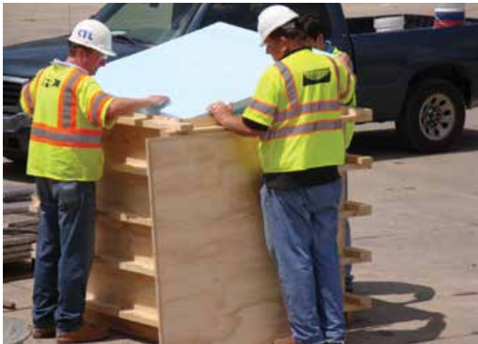
Fig. 3: After the form was filled with concrete, the top surface of the test cube was covered with three layers of 2 in. (50 mm) extruded polystyrene board insulation. The joints in the layers were staggered to prevent convective heat transfer or infiltration (refer to Fig. 1)
